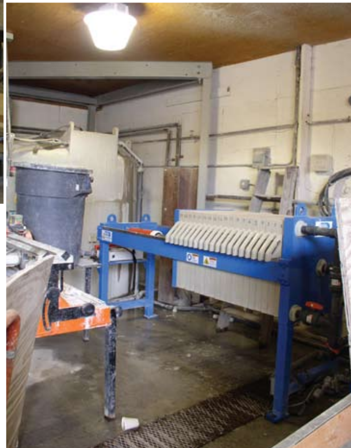
Both locations are equipped with an EnviroSystem from Water Treatment Technologies of Hampton, NH.
