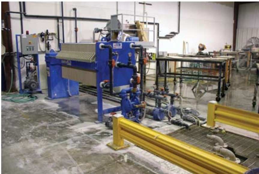
One of the most recent additions to Down East Fabrication's stone shop is a water treatment facility from Water Treatment Technologies in Hampton, NH.
